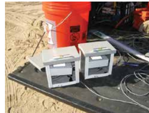
Two tilt sensors being installed on a bridge in Florida, US, by engineers from Sauls Seismic Inc.
